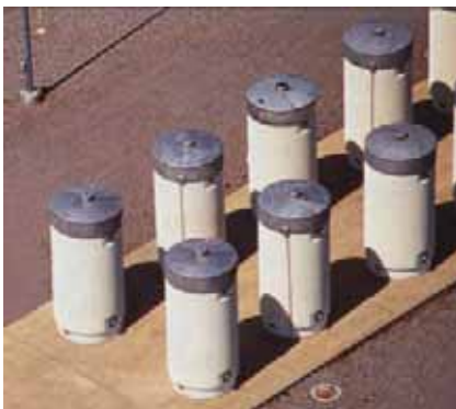
Above-ground dry cask storage.
