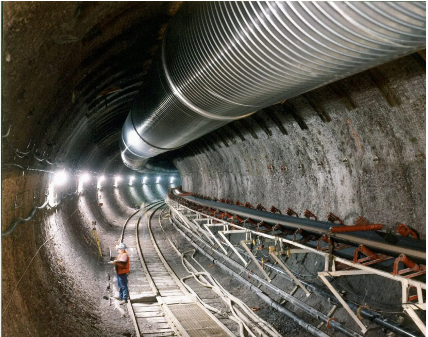
The Energy Department dug this 25-foot-diameter tunnel under Yucca Mountain to explore its potential as a nuclear waste repository. Credit: US Department of Energy
